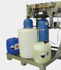
Water treatment systems
